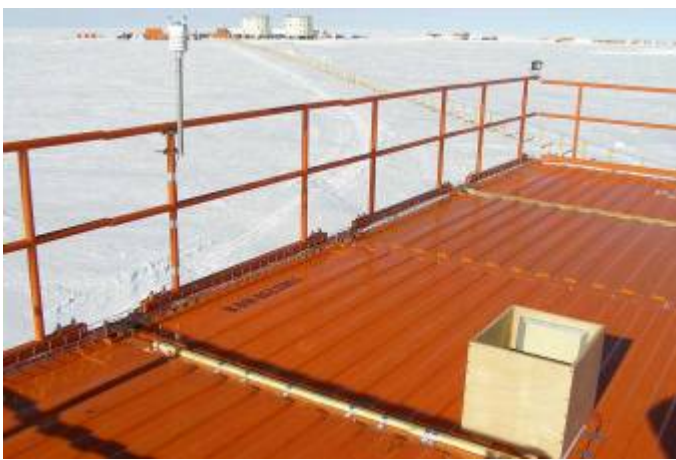
Fig. A4.4 - Roof of the Physics shelter with REFIRPAD line-of-sight and the Vaisala meteo station
